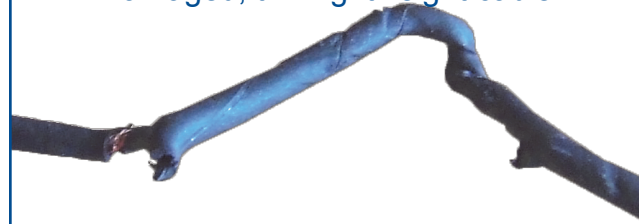
Damaged, thin lightweight cable
